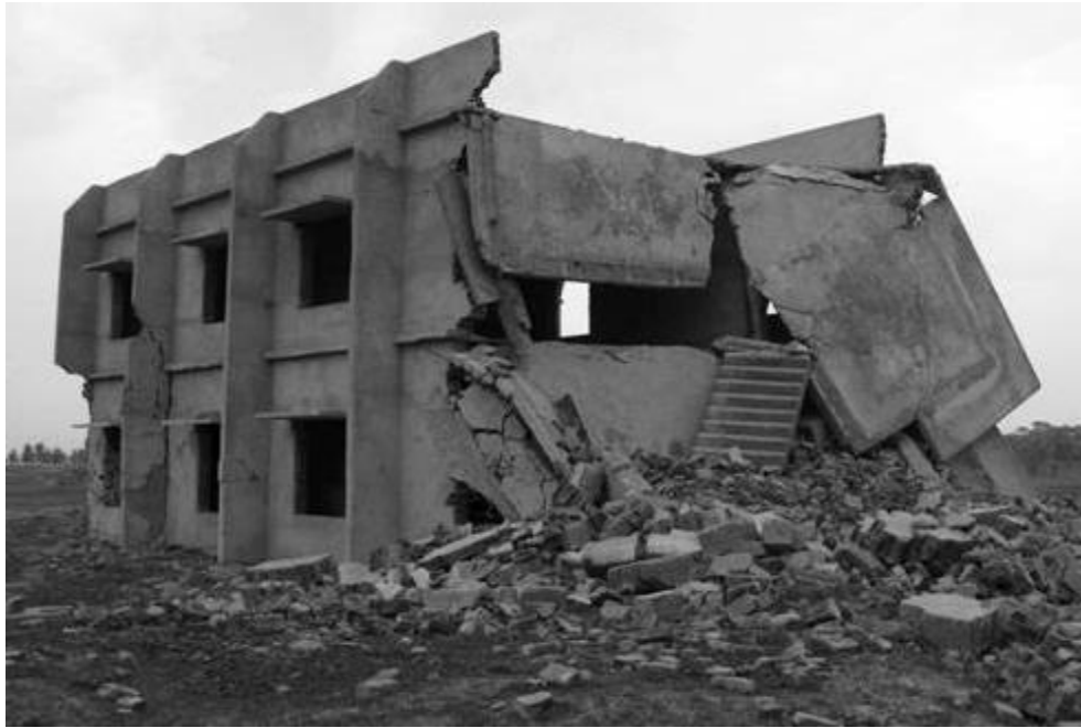
Figure 1: The damage caused to the new school building at Gosain-Pesra by a series of explosions set by Maoist fighters on April 14, 2009. © 2009 Bede Sheppard / Human Rights Watch
